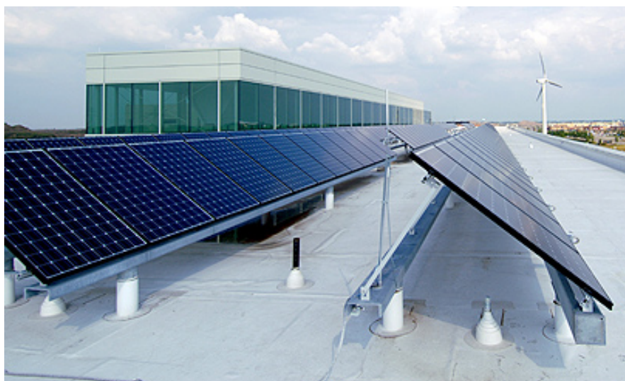
Great River Energy received CREB financing for a wind turbine and solar panels installed at its headquarters building in Maple Grove, Minn. (Photo by Great River Energy)
